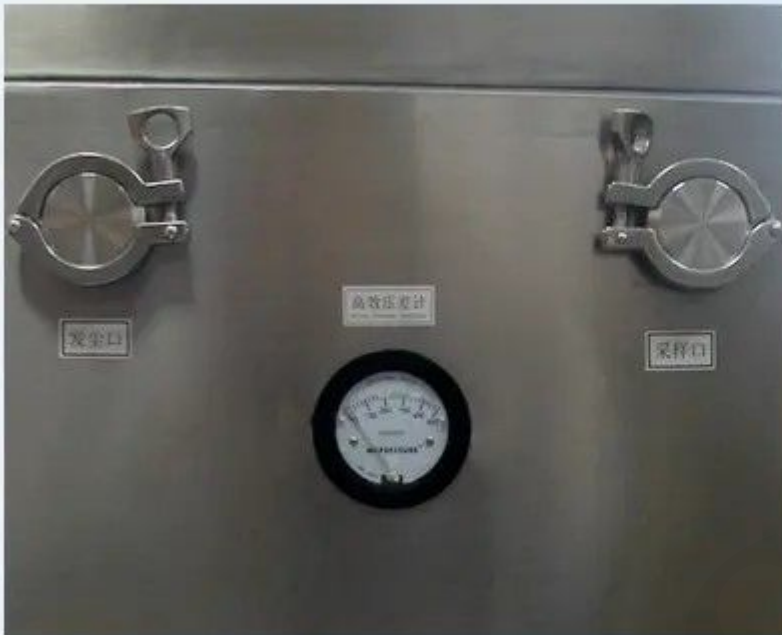
Differential pressure gauge
