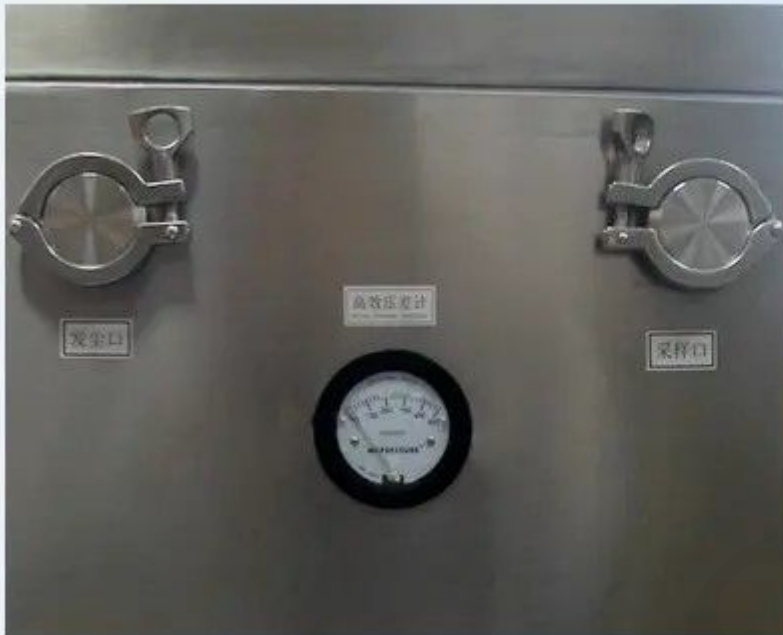
Differential pressure gauge
