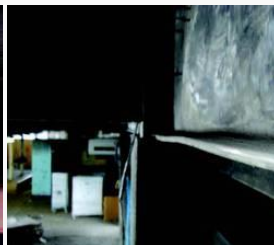
Damage of composite beam
